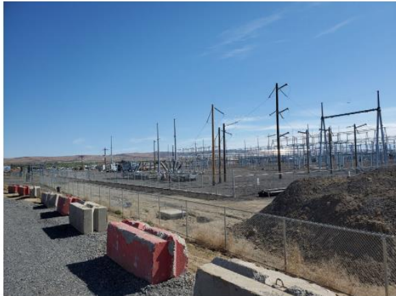
Mountain View substation
