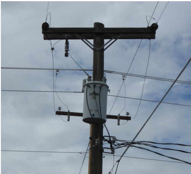
Figure 1. Typical Overhead Construction
