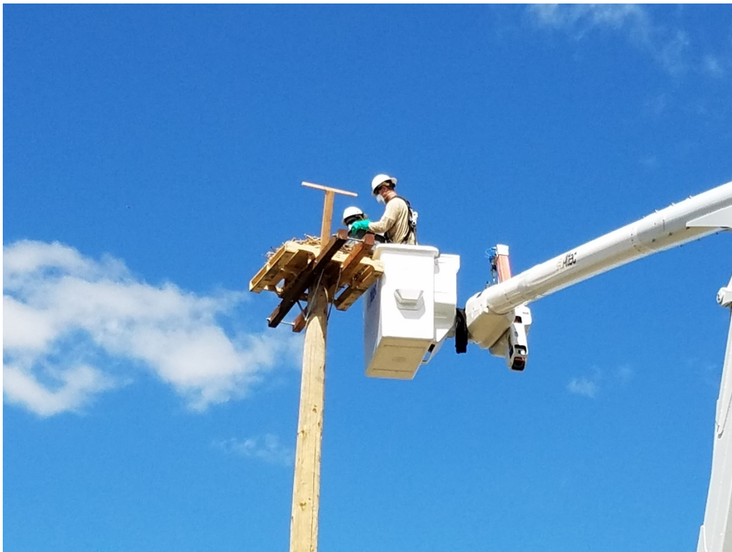
Figure 29 Raptor platform placement.
