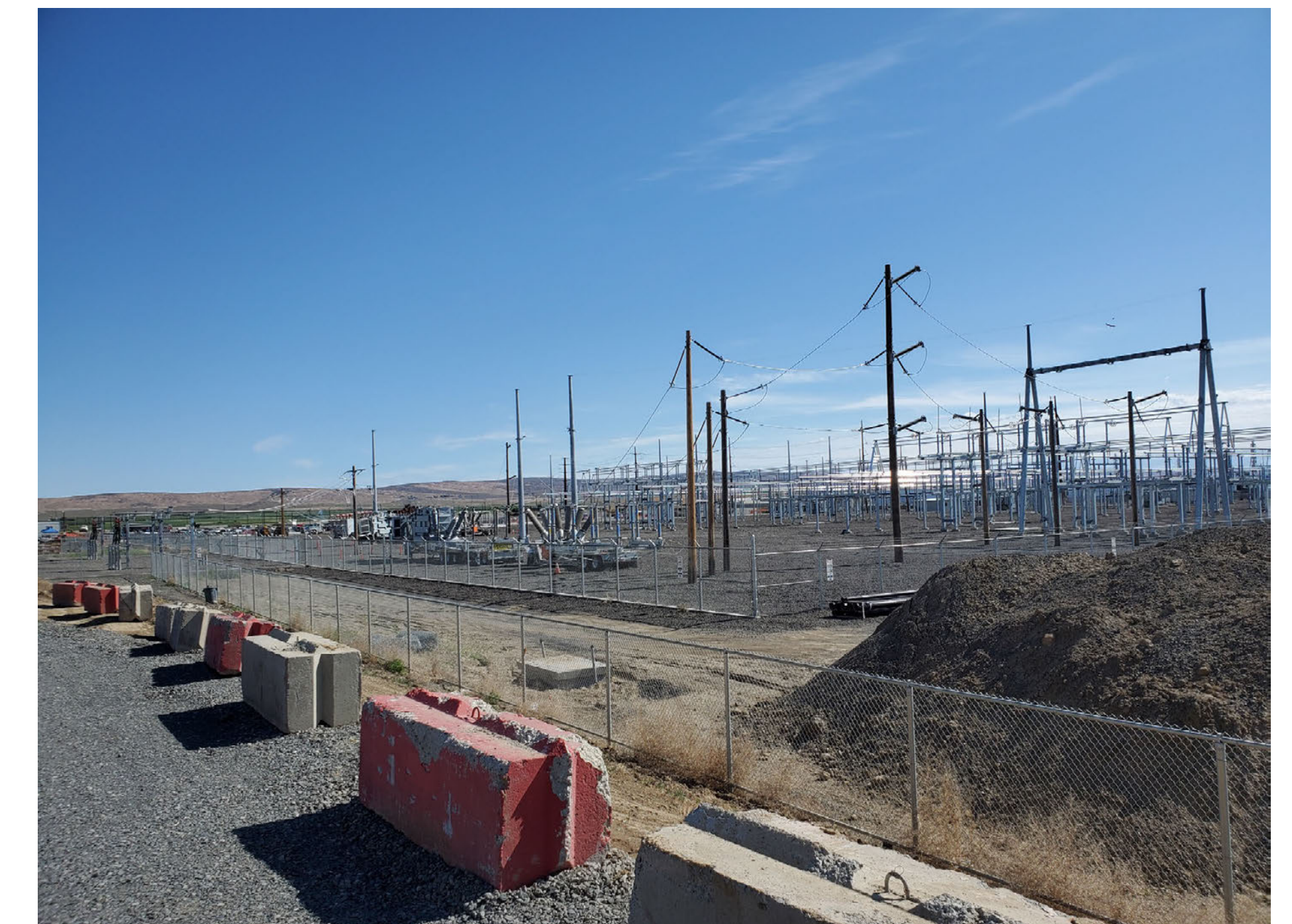
Mountain View substation
