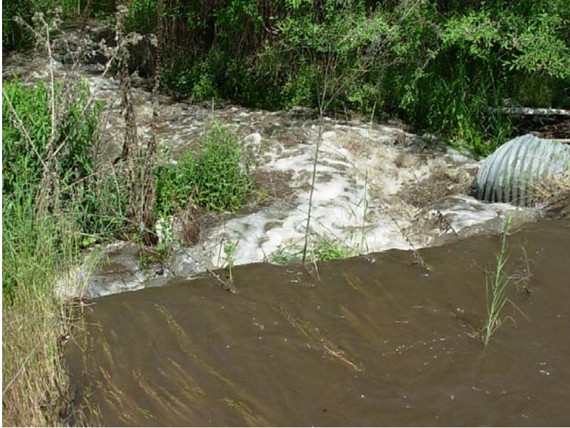
Figure 11 The undersized culvert at RM 0.35 of Antoine Creek, looking downstream, at approximately 30 cfs during spring freshet in 2006.
