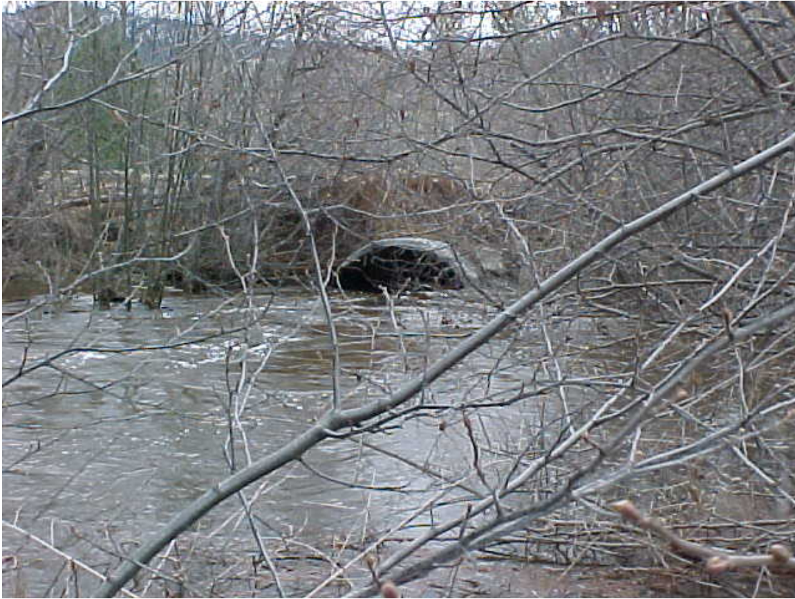
Figure 3 Culvert at RM 15, looking downstream, at approximately 150 cfs, prior to replacement.
