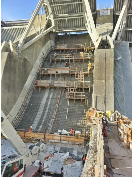
Figure 5 Priest Rapids Fish Bypass, Bay 20 Apron and Ogee Concrete Curing and Preparation Work. December 2013.
