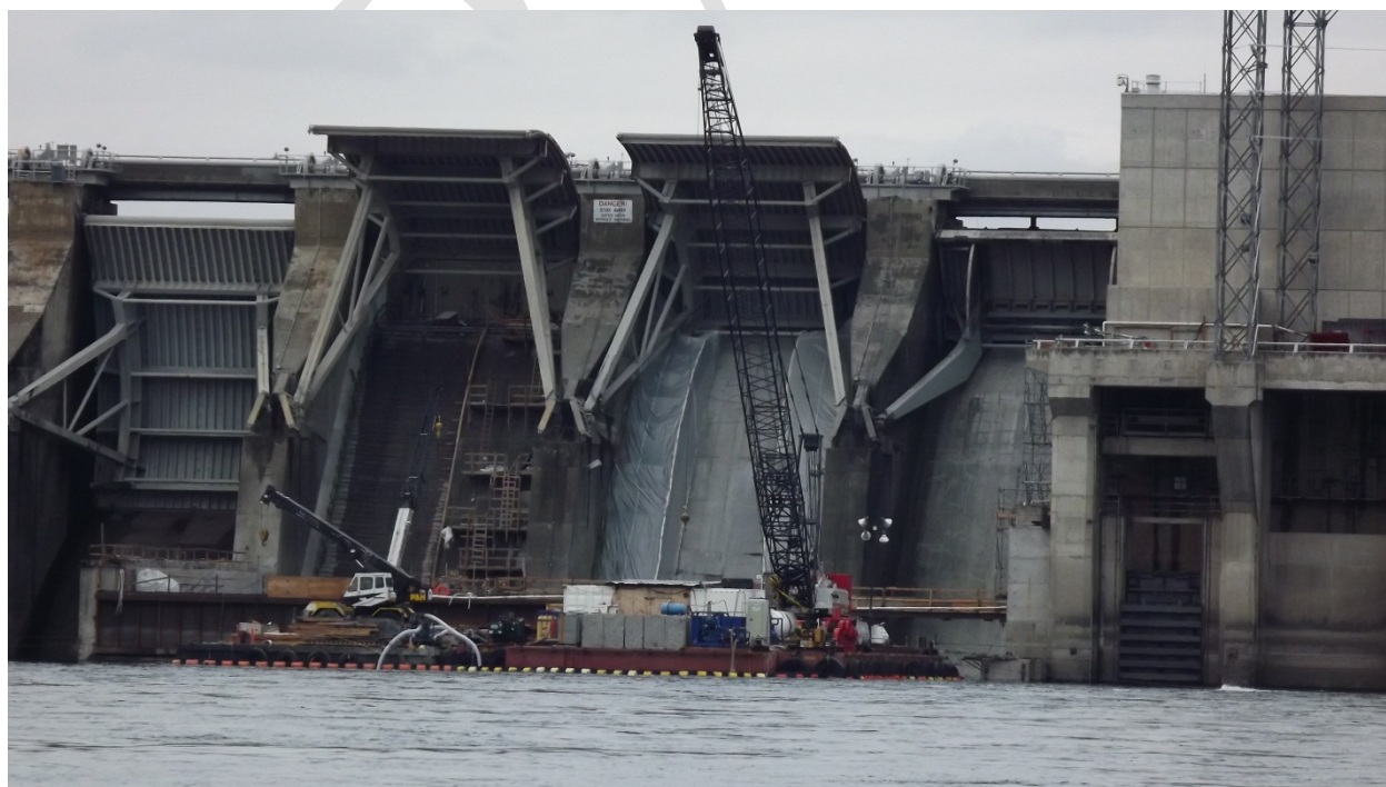
Figure 4 Priest Rapids Fish Bypass Construction Activities. Looking Upstream at Gate(s) and Spillway Improvements, December 2013.
