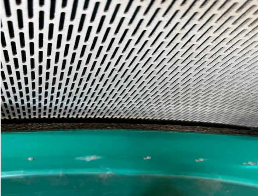
Figure 1. Gap at the base of the side screen of the overflow pump.
